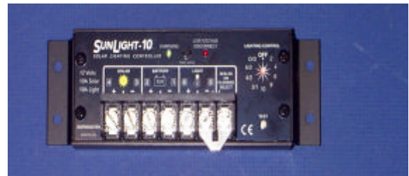
Figure 2-6. PV lighting system controller (Morningstar).
