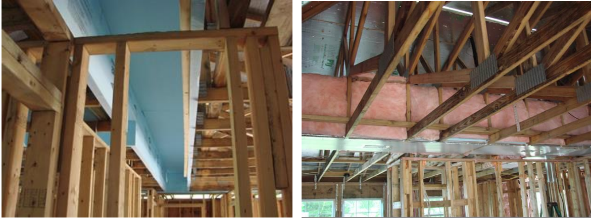
Figure 10. SEVHFH lined the inside of their fur up chase with rigid foam insulation, and then wrapped the top and sides with batt insulation for a total of R-33.
