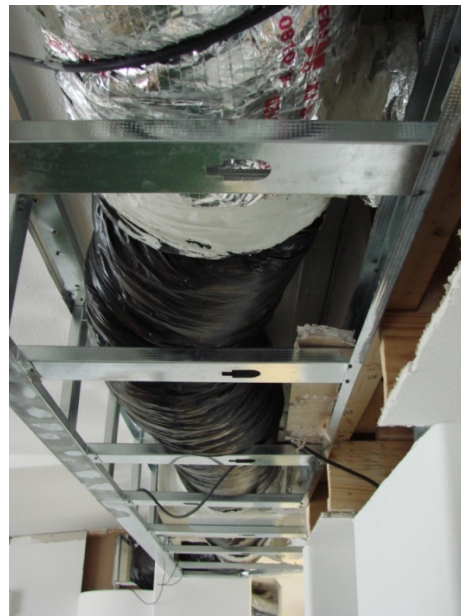
Figure 6 MHLab soffit duct (supply side).
