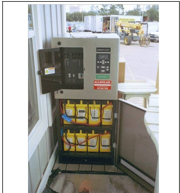
Figure 5 – Inverter system with battery backup
