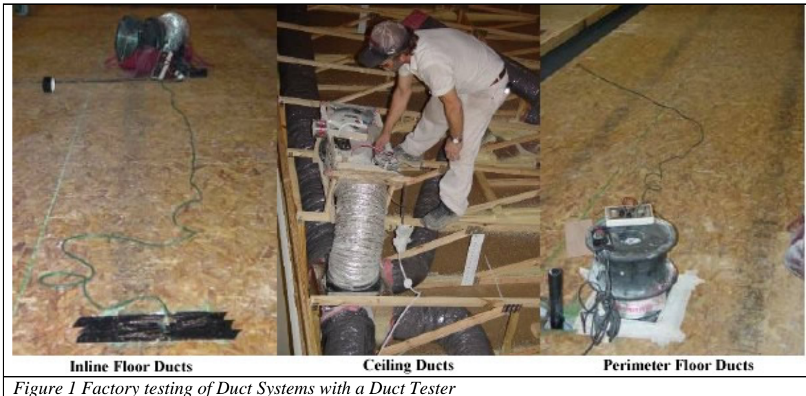
Figure 1 Factory testing of Duct Systems with a Duct Tester
