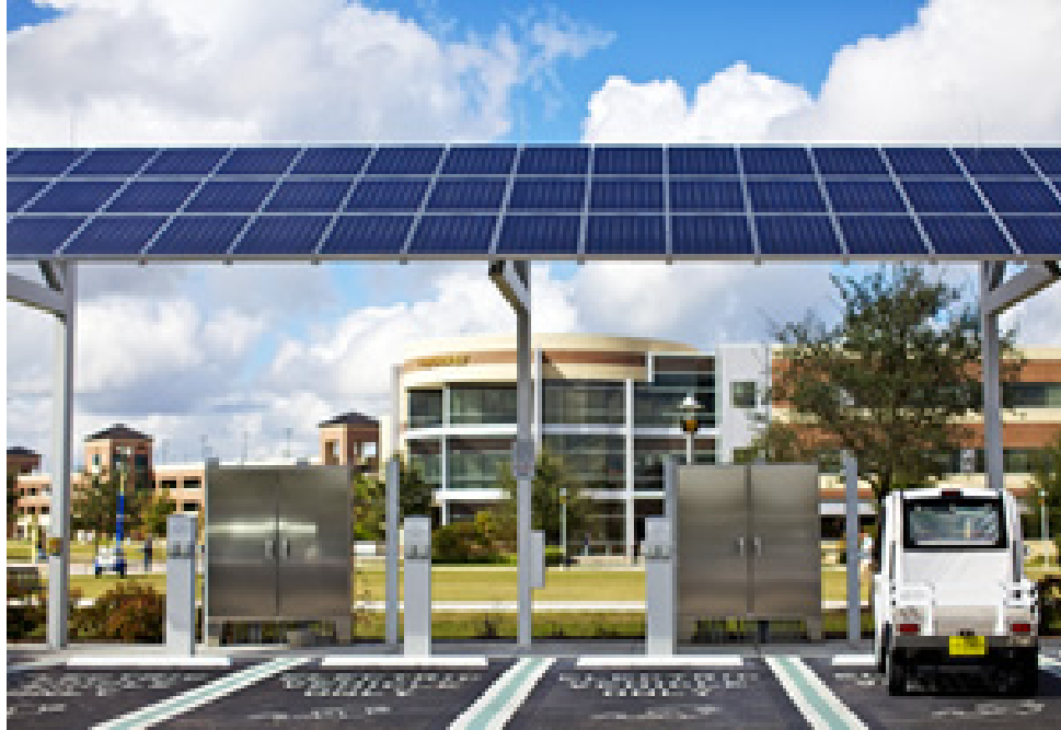
Figure 1. Electric vehicle charger on UCF campus with PV power assist. Photo: Enrico Sacchetti
