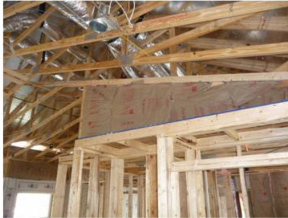
Figure 10. Batt insulation installed to backer board from Figure 9; six-sided sealing of cavity is provided by backer, facing drywall (yet to be installed), and framing members
