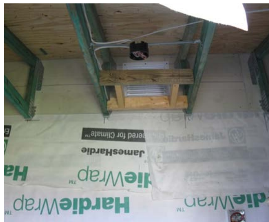
Figure 12. Closet under construction. Grille on back wall connects attic space of closet to vented attic of house through gable end. Rough framing can be seen for grille in closet ceiling that will complete connection between closet and attic.
