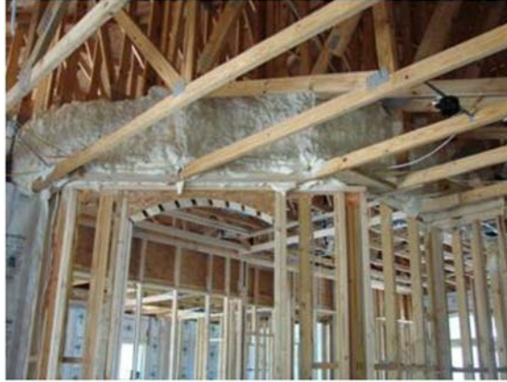
Figure 7. Foam applied to knee wall in attic where ceiling heights transition from 8 to 10 ft
