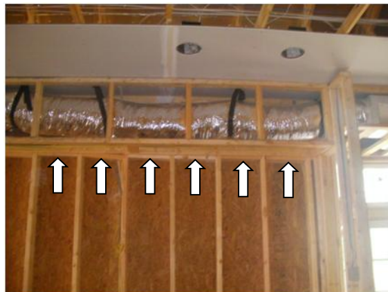
Figure 5. Arrows point to code-required fire blocking under chase, preventing insulation from being easily installed behind duct. Correction involves re-sequencing so insulation can be installed in this area prior to duct.
