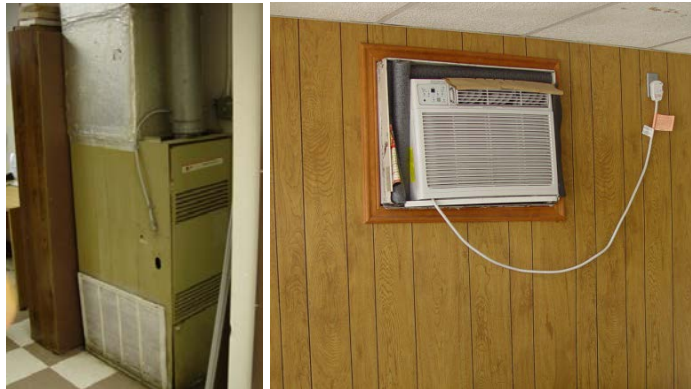
Figure 5. Natural gas furnace (left); window AC unit, fitted into rough opening with cardboard and foam (right)
