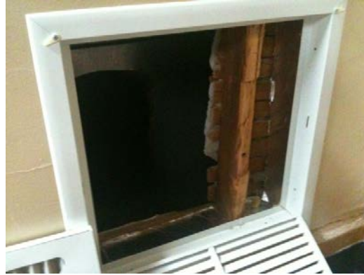
Figure 13. Post-retrofit, researchers observed an airflow pathway from a large open wall cavity between the AHU and the filter grille
