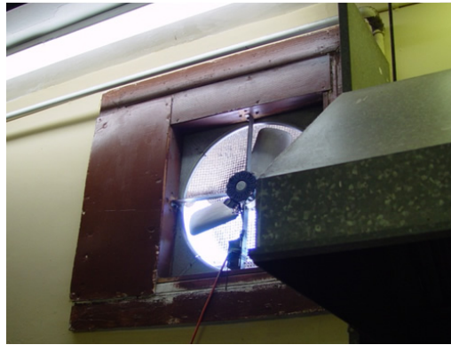
Figure 4. One of two through-the-wall exhaust fans ventilating the kitchen
