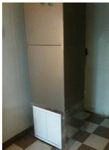
Figure 14. Post-retrofit ground floor, SEER 15 heat pump AHU
