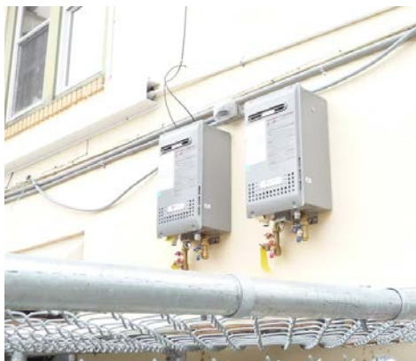
Figure 15. Two externally mounted gas tankless water heaters
