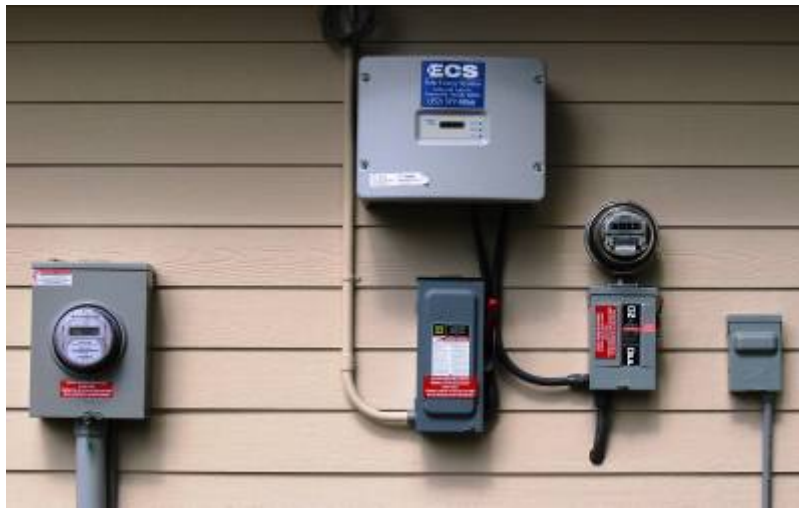
Figure 8. Inverter and electrical interface at NZEH house.
