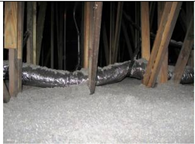
Figure 5. R-30 cellulose attic insulation, radiant barrier vented attic and R-6 flex duct.
