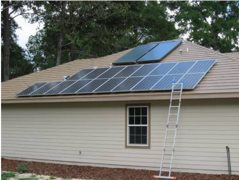
Figure 10. Closeup of 3.1 kW PV system and 80 ft 2 solar water heating system.
