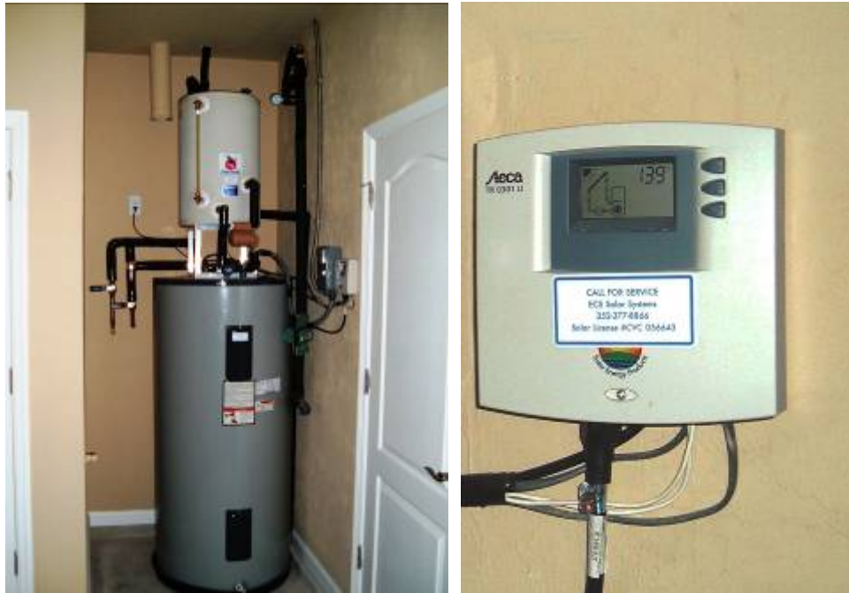
Figure 16. 120 gallon solar water tank with monitor showing system function.
