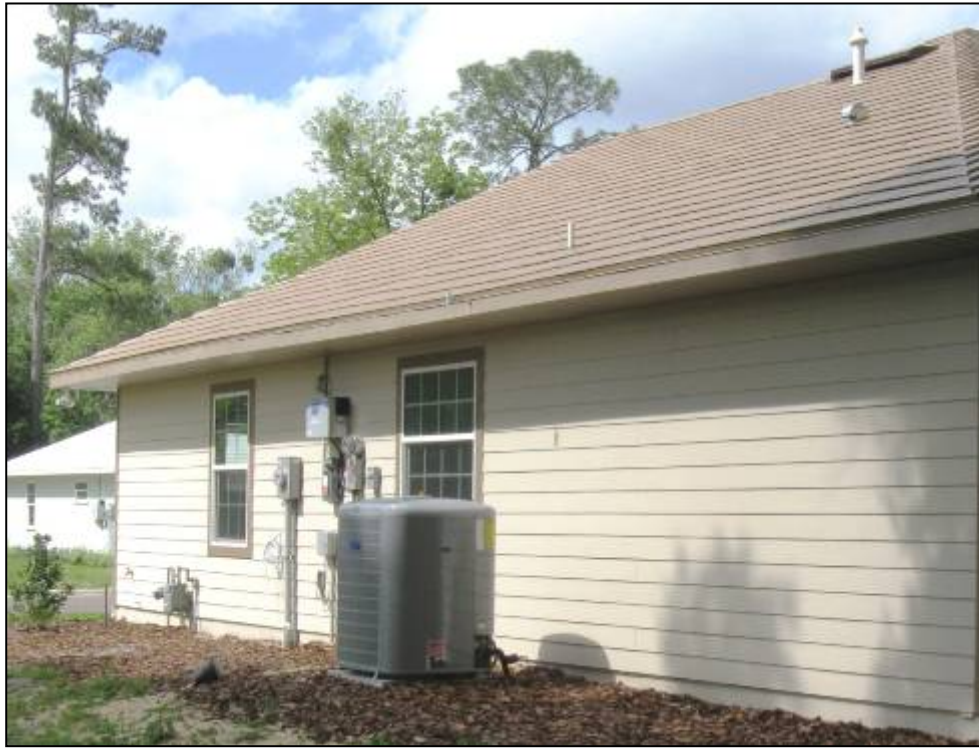
Figure 6. SEER 19 AC system on east side of home with grid-tied SMA inverter in background.
