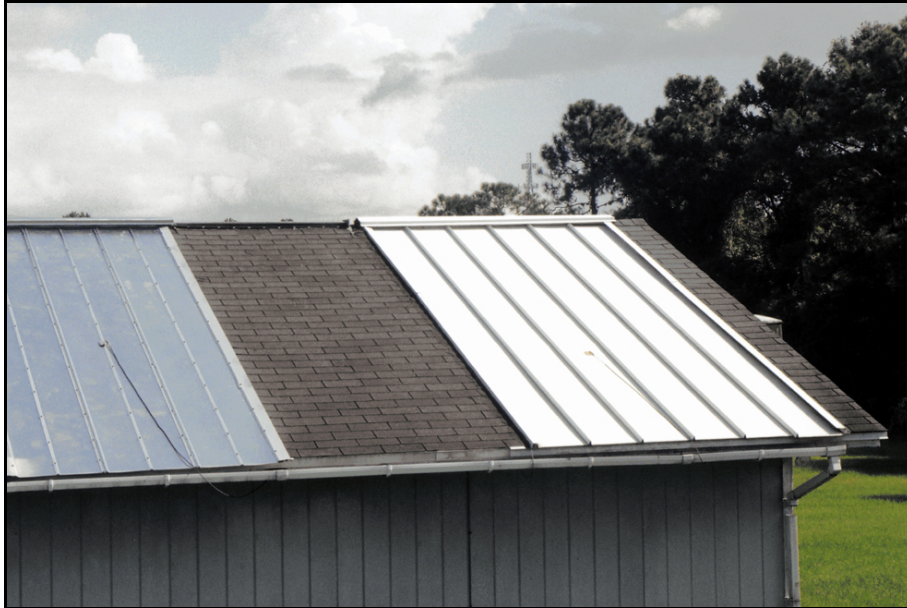
Figure 1. White standing seam metal roof on the right at the Flexible Roof Facility (FRF) used to evaluate NightCool potential.
