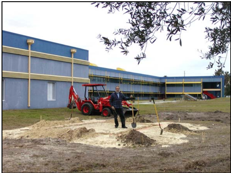
Figure 20. The two 10 x 16' small experimental night cool buildings are being constructed 20 ft. south of the Building Science Lab.
